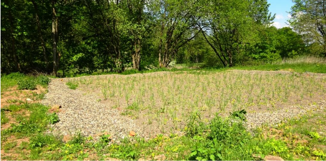
Picture: Reed bed sewage treatment field
