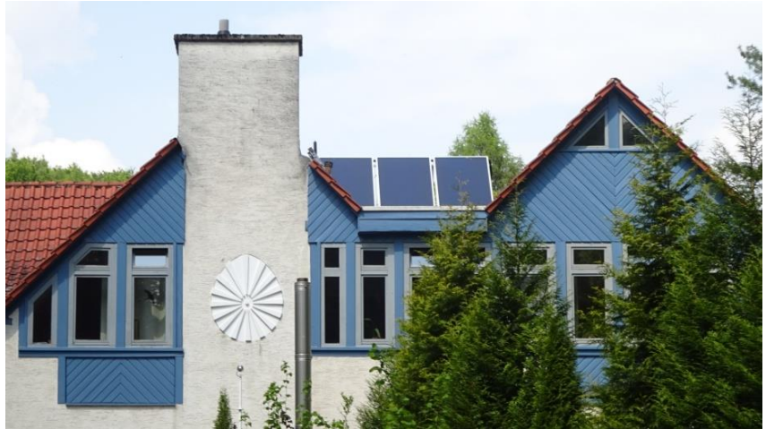
Picture: solar plate collectors on the roof of Moringen
